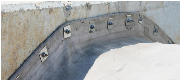
CC fixed to concrete headwall
