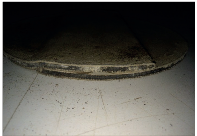
Figure 10. CC5-2 joint after the test, no root penetration
