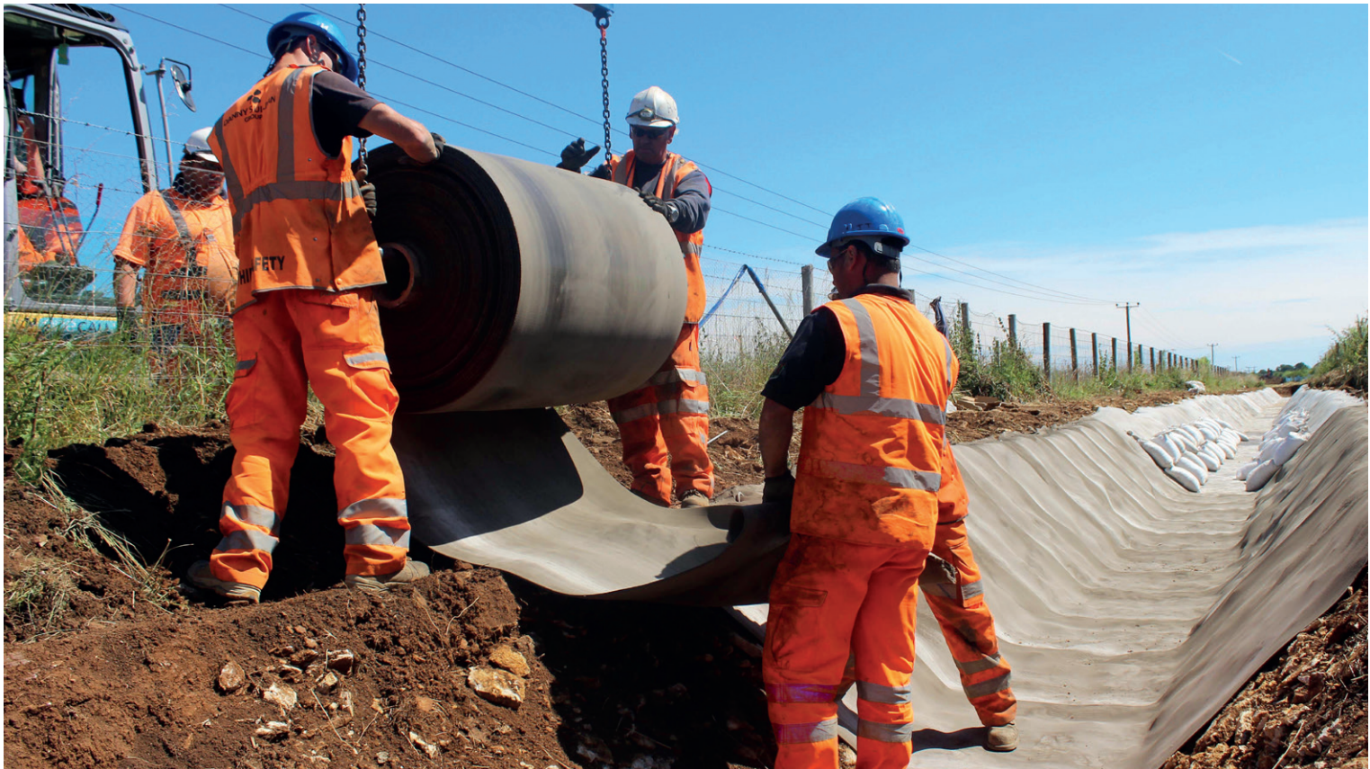
CC being used as an alternative to poured (in-situ) concrete for channel lining.
